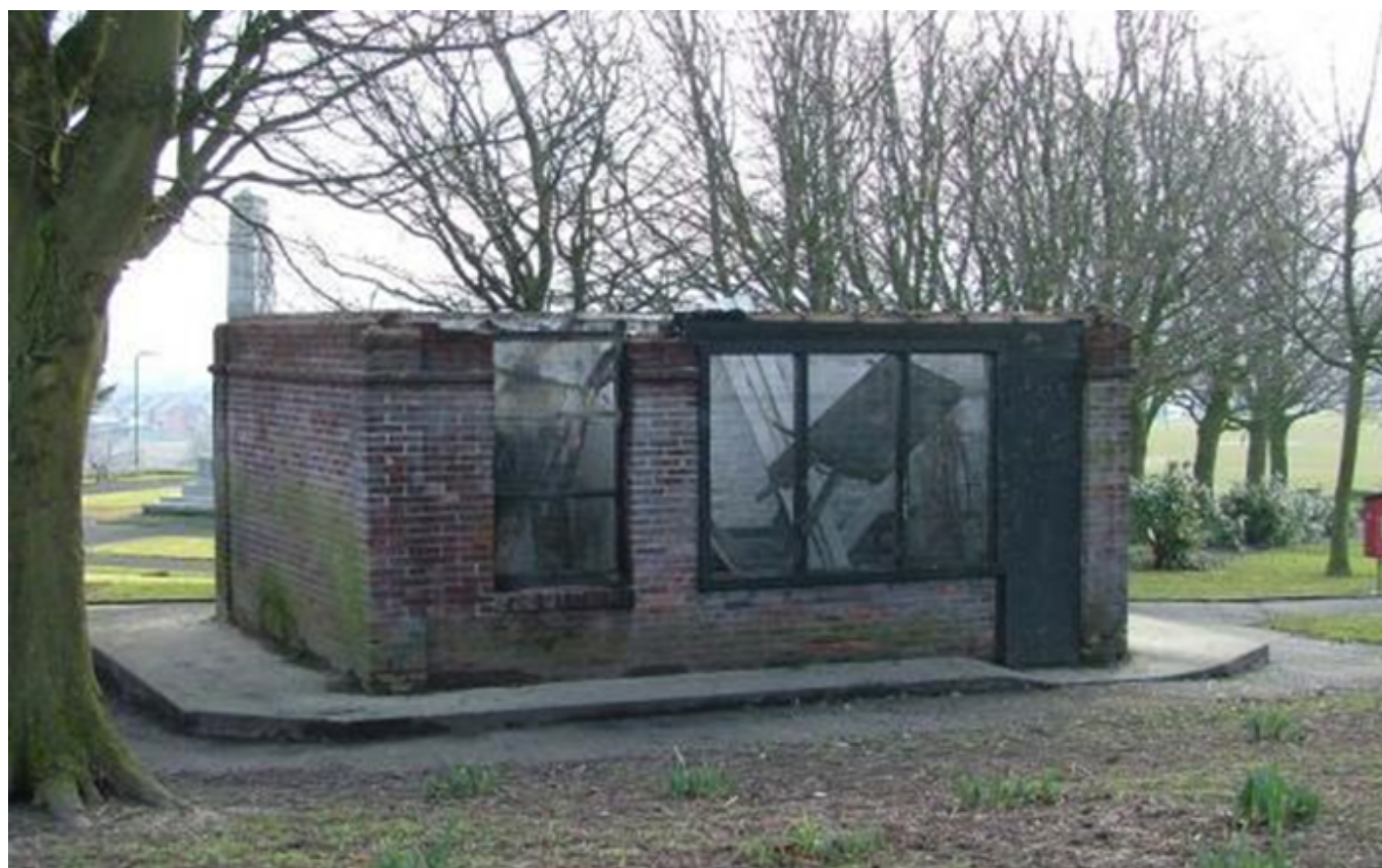
The budgie hut after a fire, 2006
